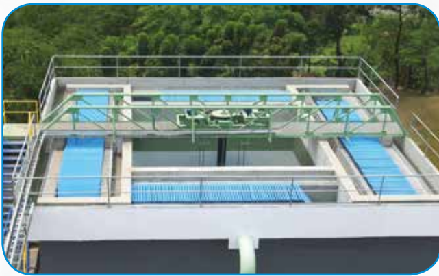
INDION Ultra High Rate Solids Contact Clarifier (UHRSCC)
